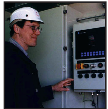
Alan Wassens, Maple Lodge Engineering/Services Manager, inspects the Allen-Bradley control panel. Wassens was a strong advocate of cogeneration for the plant. "It was a matter of finding the right fit," he says, "and rationalizing the financial investment."
